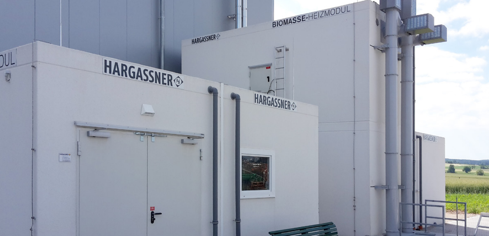
Schwandner Logistik in Pfreimd, 2 x 150 kW Hackgut
